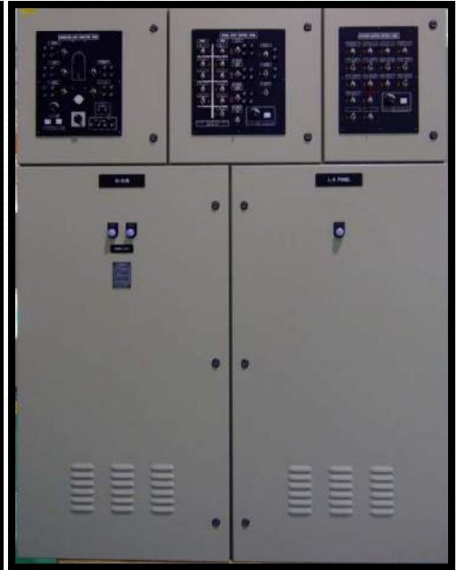
[Group Control Panel]
