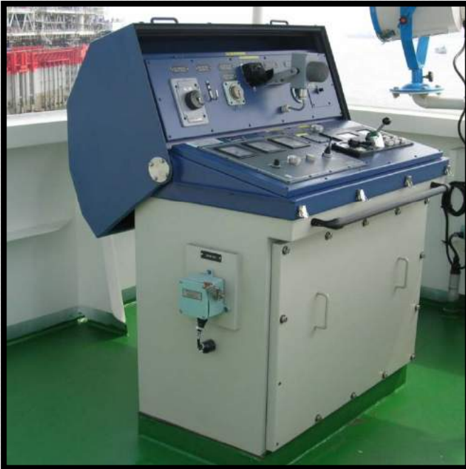
[Bridge Wing Control Panel]
