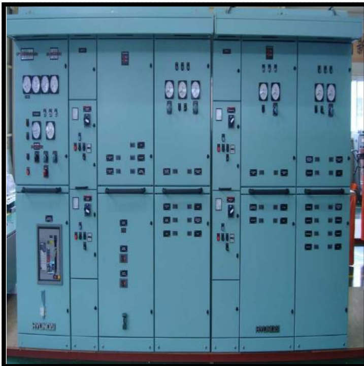
[Motor Control Center]
