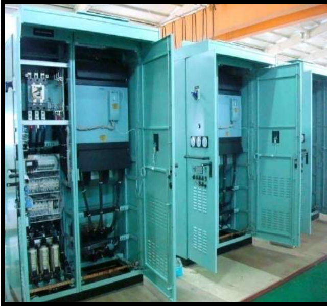
[Vacon Inverter Panel]
