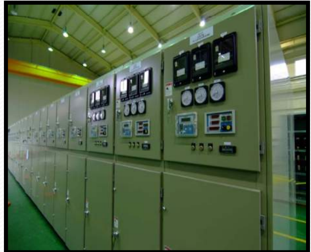
[ High Voltage Switchgear]
