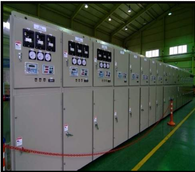
[ LV TR Switchgear ]
