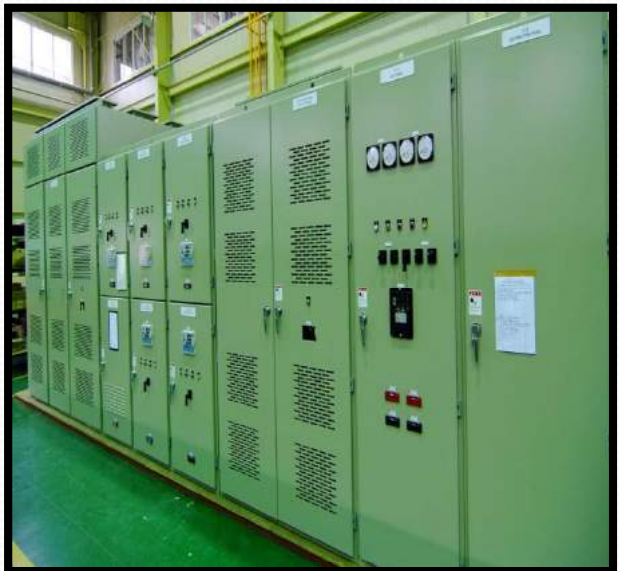
[ High Voltage Switchgear ]
