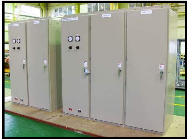
[ UPS Power Dist board]
